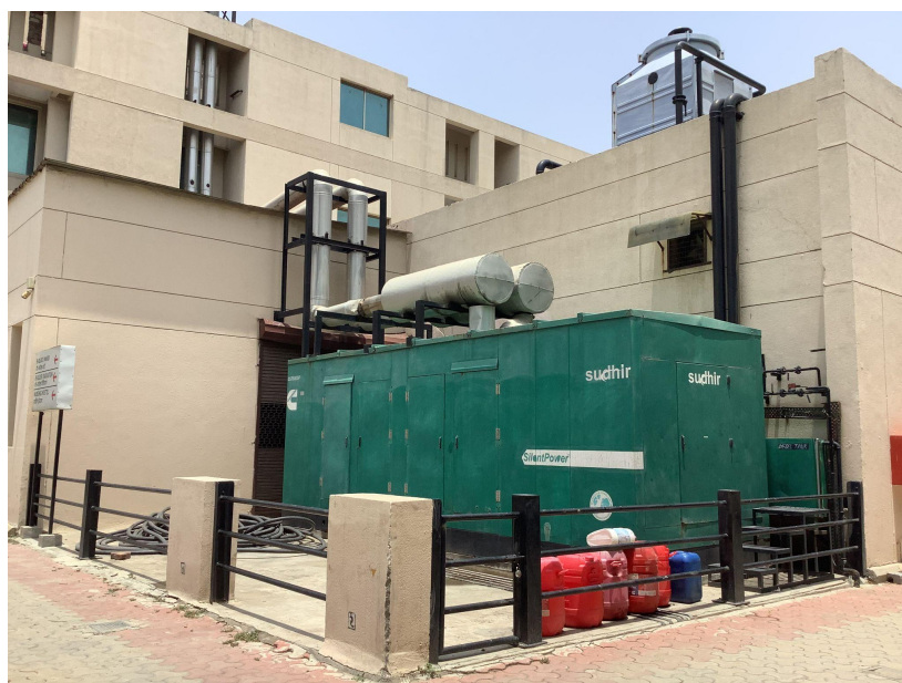
Fig- 2 DG Set of 750 KVA capacity is installed at the site for emergency power backup. At present, the DG set is not being used, and the site is operating on regular electricity supply.
